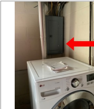
Electrical panel did not have proper clearance in front.
